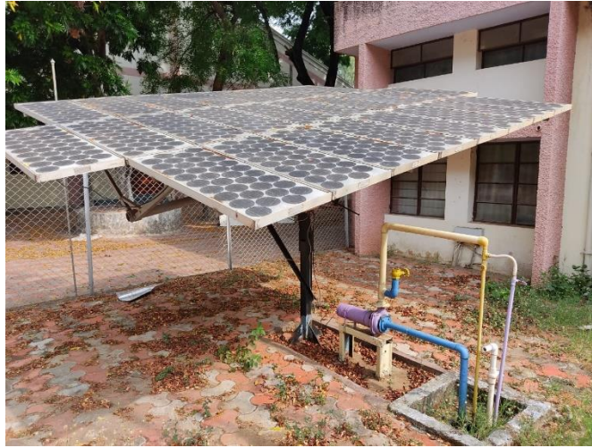
Fig. 6 Solar PV System
